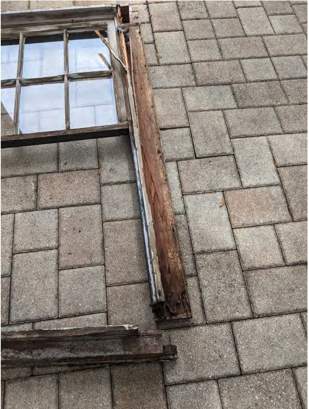
Current window is too rotten to re-install
