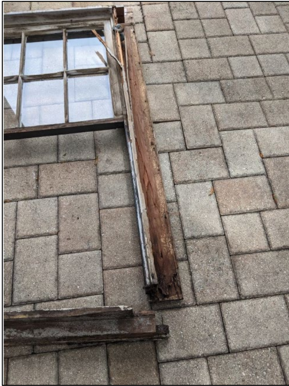
Figure 6: Deteriorated historic window (applicant photo)
